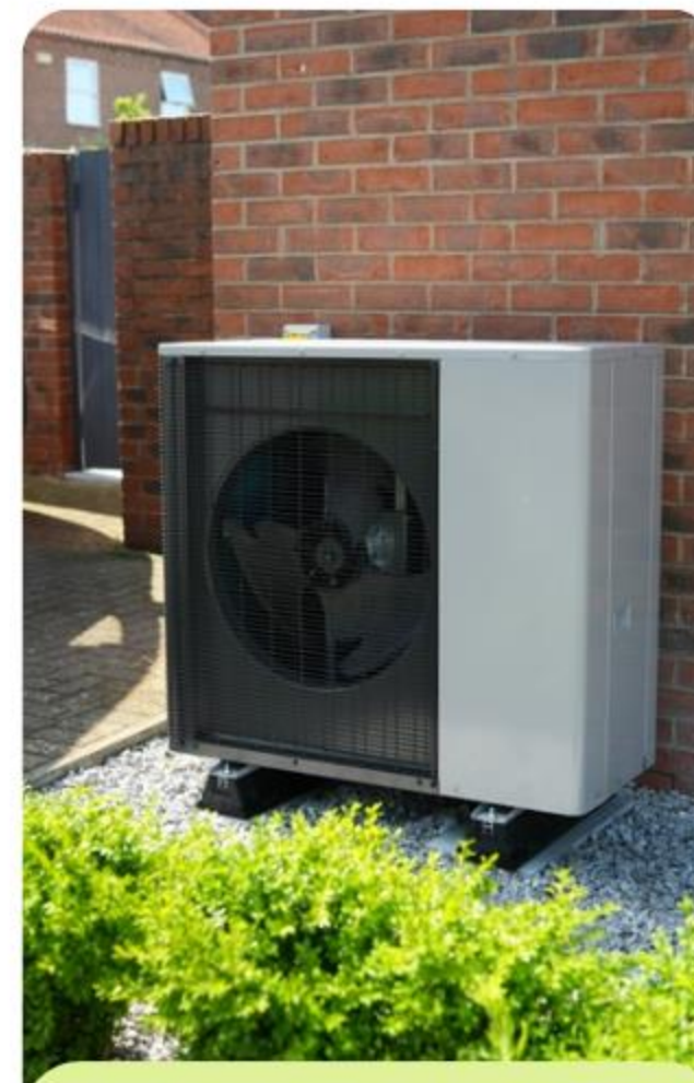
Air-to-air heat pump Administrative building Carna Carpatica
